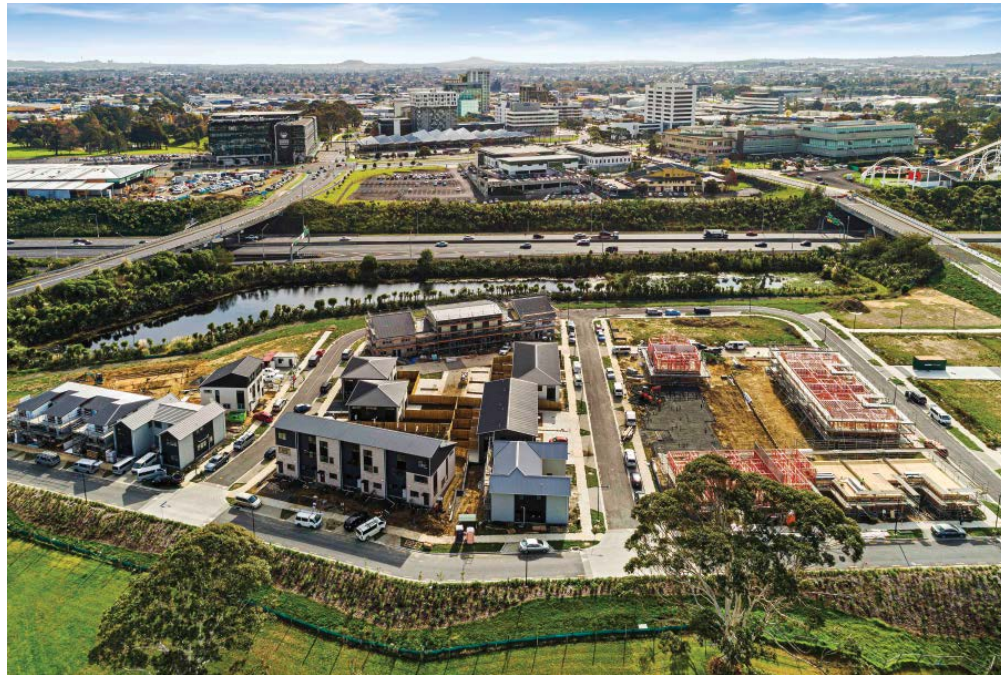
190 homes at Puhinui Park are under construction by the consortium made up of the New Zealand Housing Foundation, Te Tumu Kāinga, and CORT.
